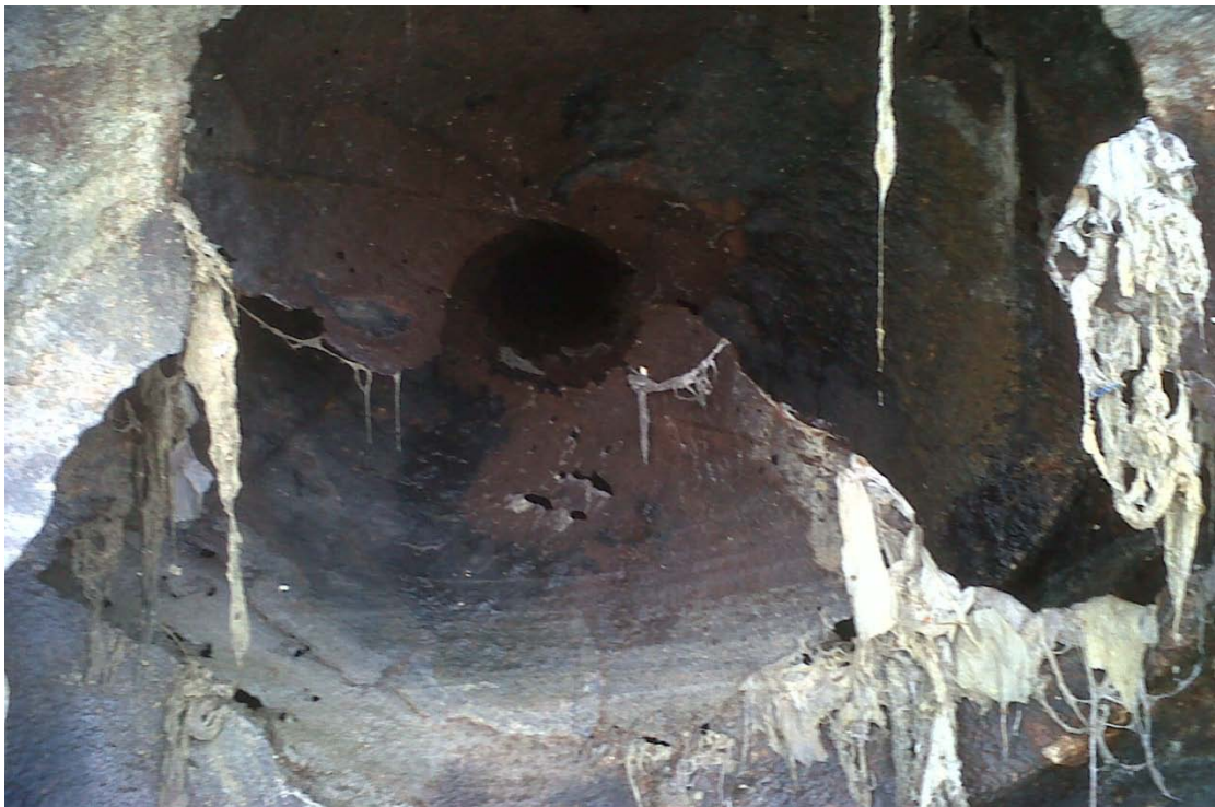
Interior flights missing 2 to 3 feet inside pump #3
