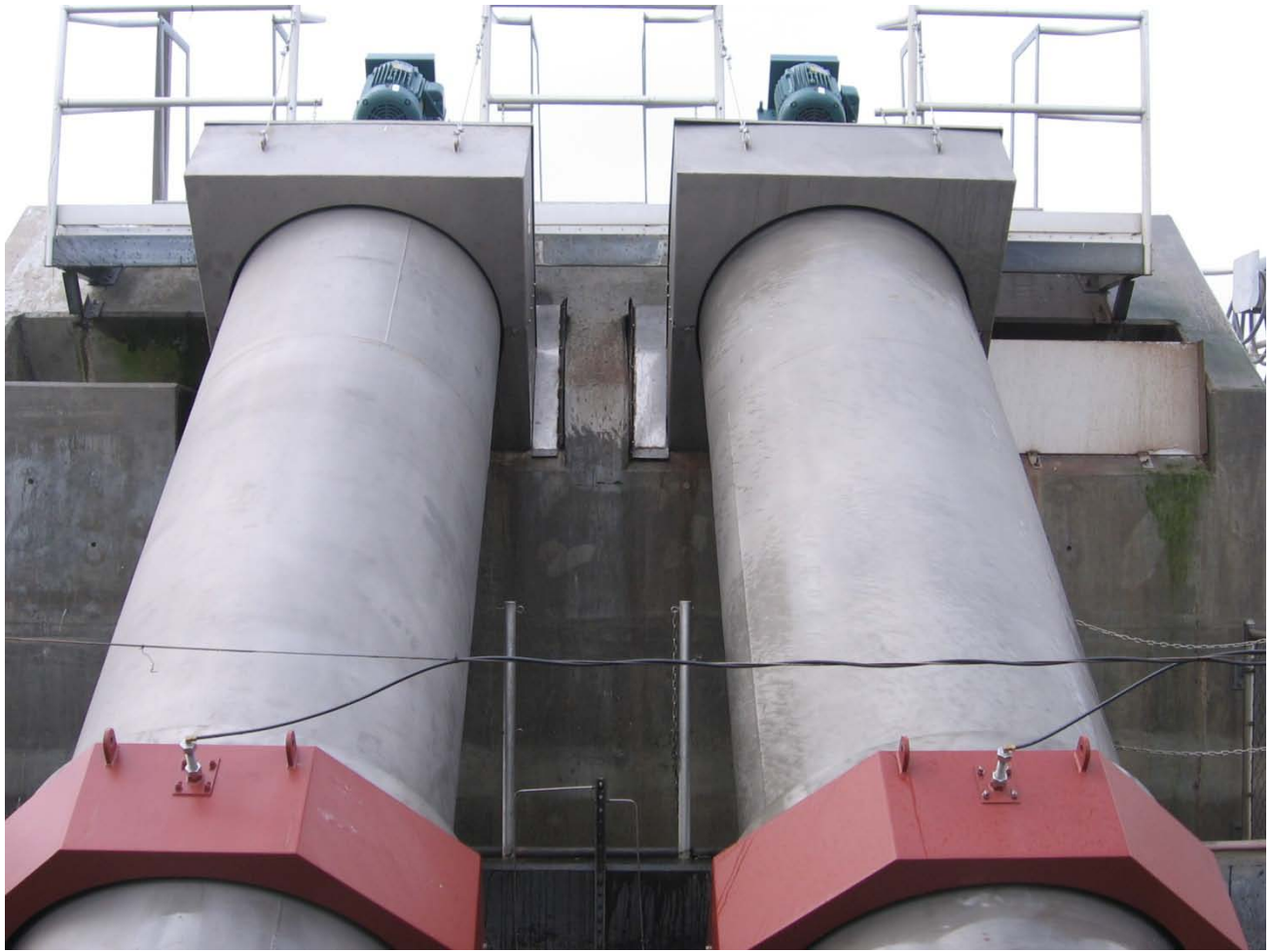
Two New Return Activated Sludge (RAS) pumps.
