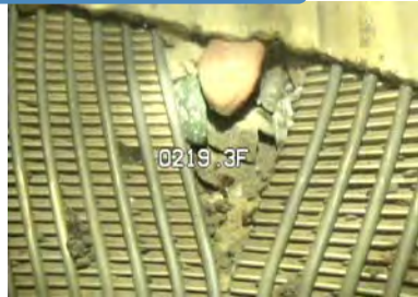
Torn Well Screen
