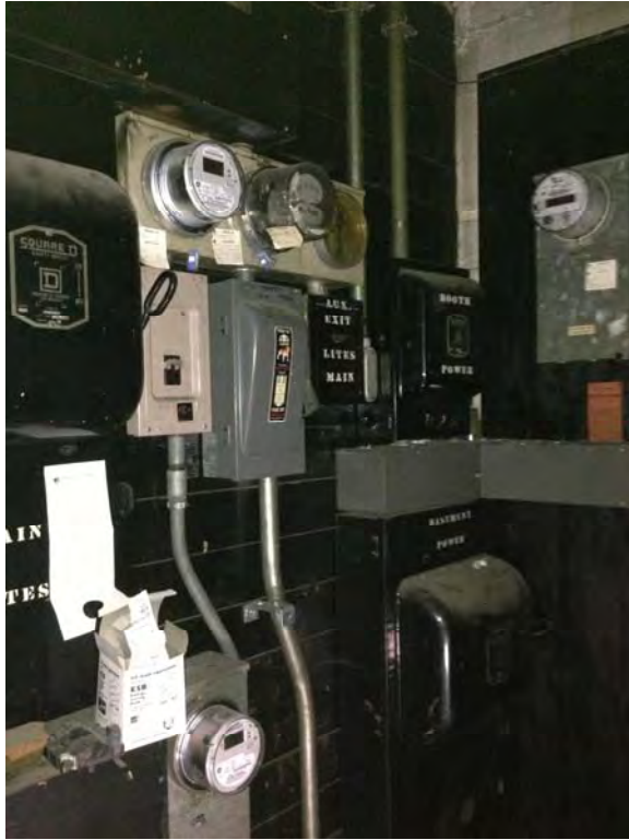
84. Main Service Feeding Small Theatres
