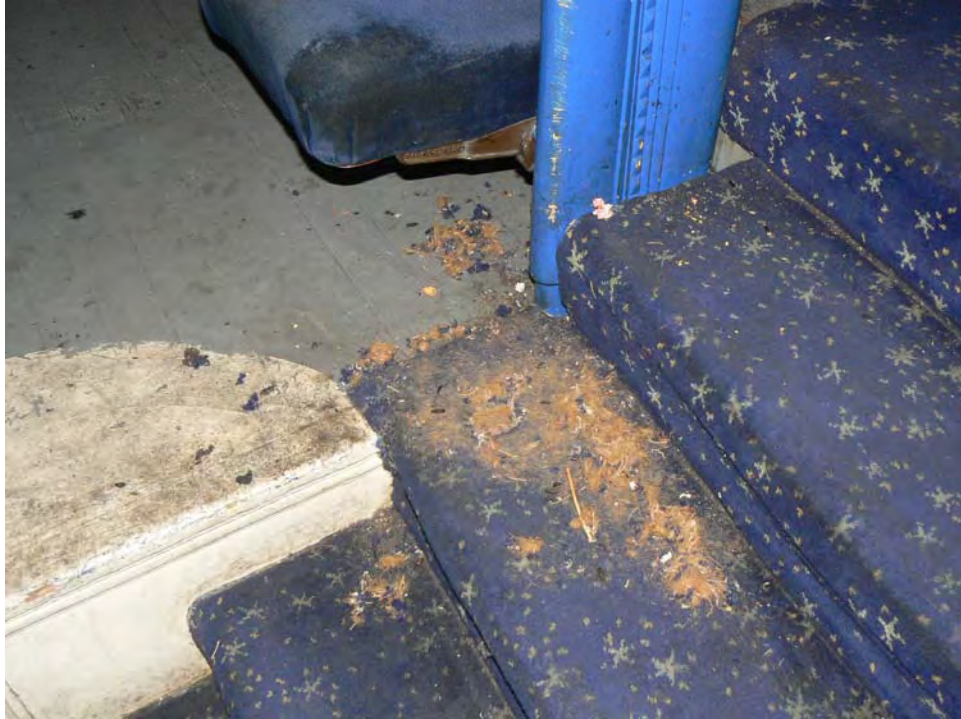
63. Auditorium - Floor Condition
