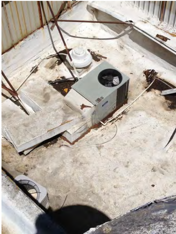
79. Roof - Existing HVAC Unit for West Theatre
