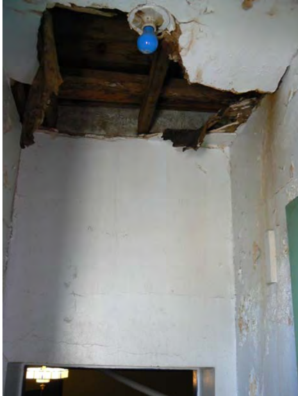
70. Projection Room - Ceiling Condition
