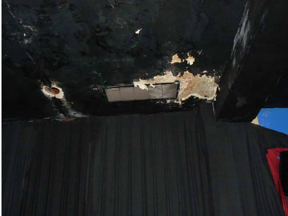
31. East Theatre - Ceiling Condition at Mechanical Grille
