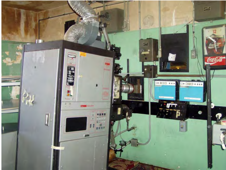
71. Projection Room Equipment
