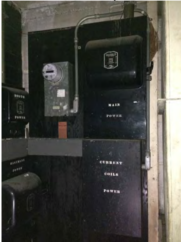
83. Main Service Feeding Main Auditorium
