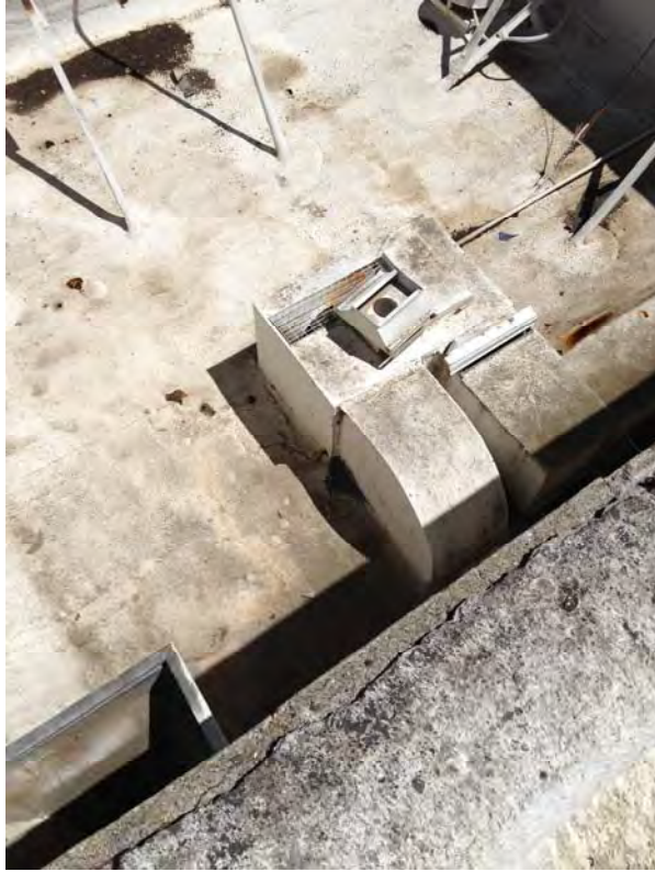
78. Roof - Existing HVAC Unit for East Theatre
