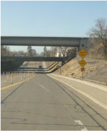
Underpasses and other low points can be subject to localized flooding during periods of heavy rainfall.
