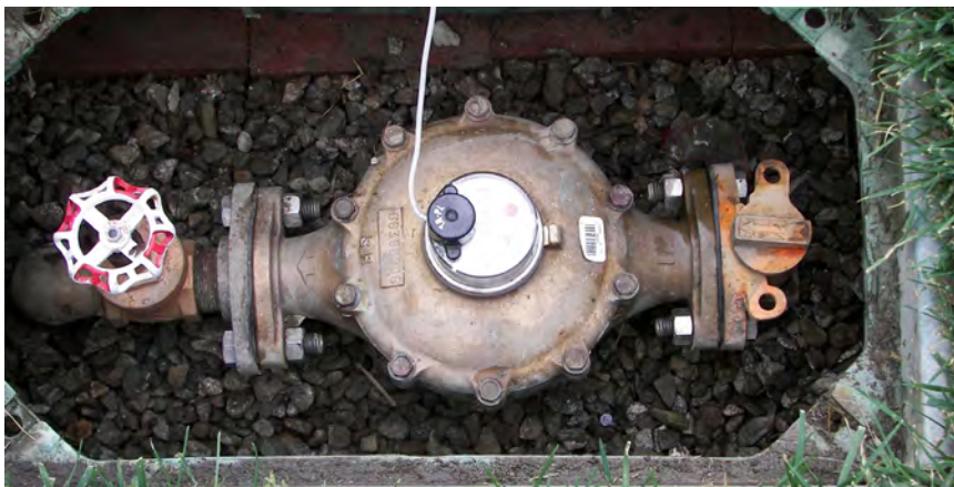
In 2011, water meters were installed at every home in Woodland in order to comply with State law. Water customers are now billed based on how much water they use, which is anticipated to reduce demand and help conserve water supplies.
