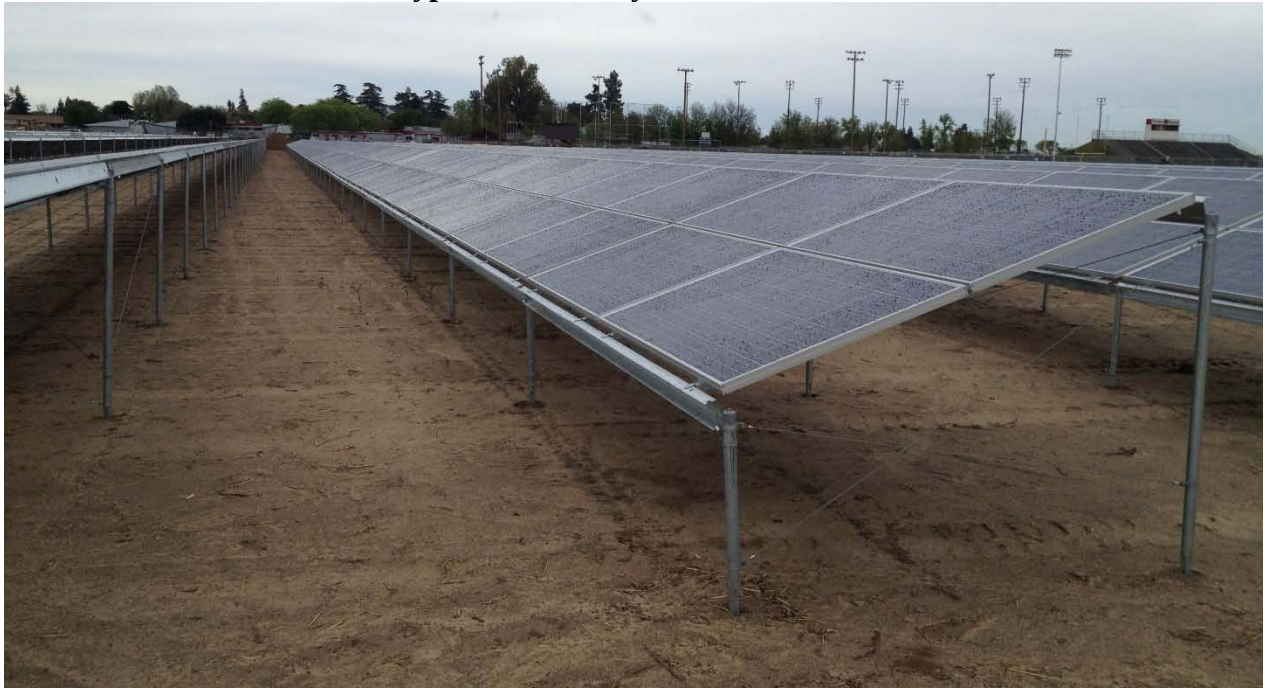
Figure 3 Typical Stationary Ground Mount
