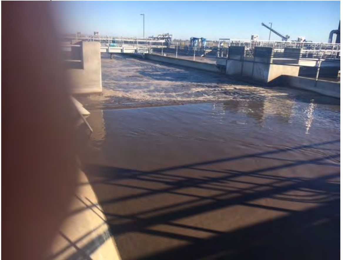
Basin 3 in operation
