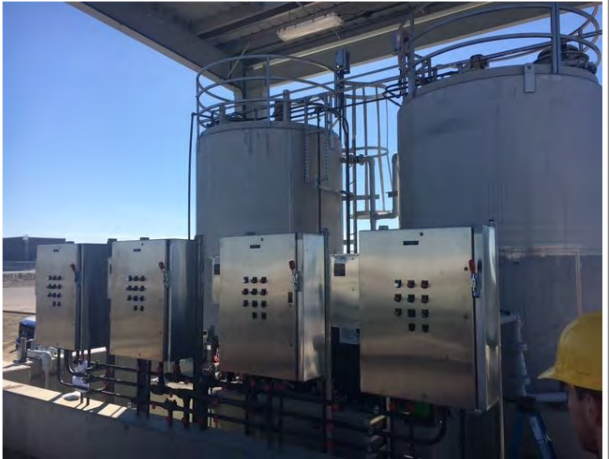
Alkalinity tanks and controlsMissyisno1
