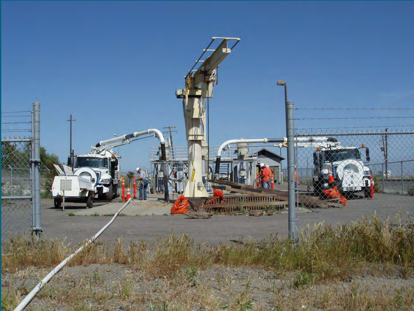
E. Main Lift Station
