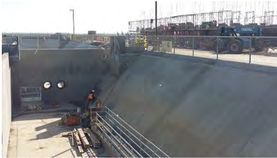
Modified oxidation ditch with beginning of blower building behind
