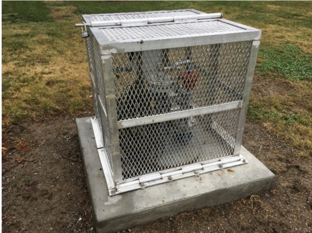
Monitoring wellhead in cage
