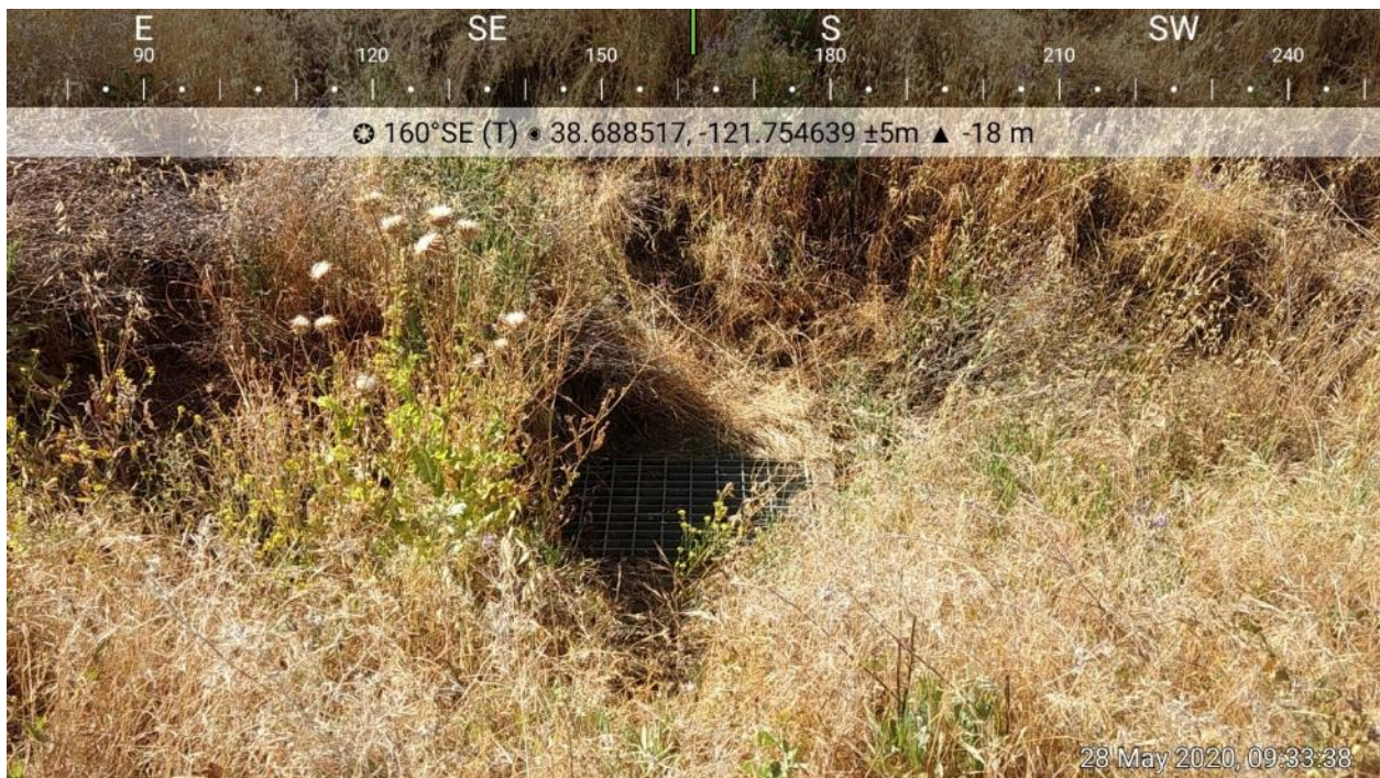
Photo 6: The storm drain inlet present at the eastern end of the upland drainage swale in the southeastern corner of the Project site, looking south.
