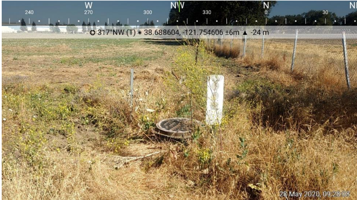
Photo 7: An example of one of the three storm drain inlets present in the Project site along the eastern border, looking northwest.
