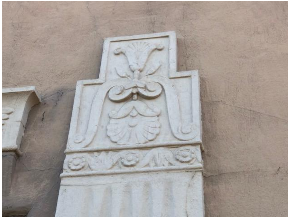
Photograph 12: Close-up view of the capital atop the pilasters representing a stylized lotus flower.
