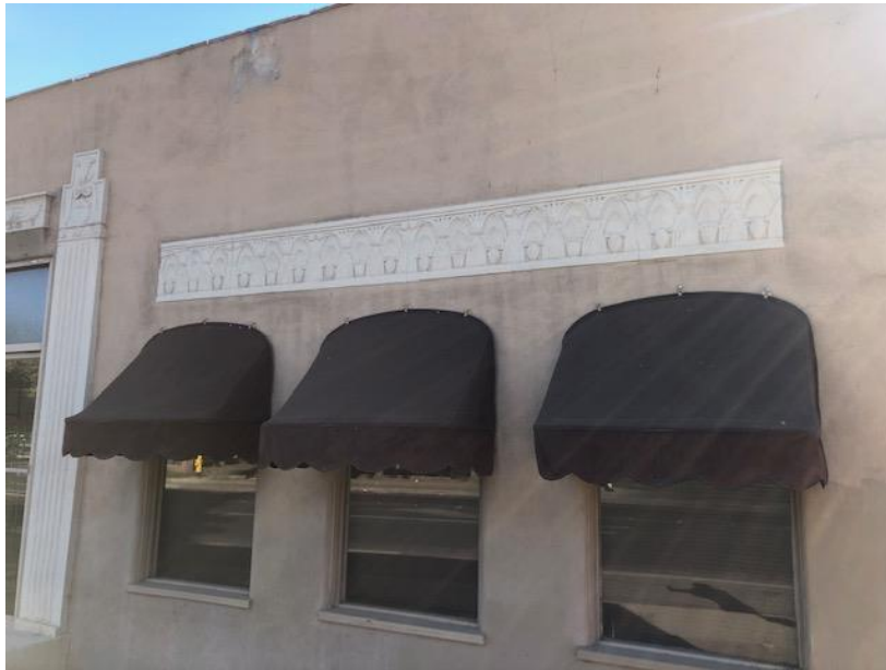
Photograph 9: View of the Art Deco stylized Egyptian Revival frieze above the west elevation windows.
