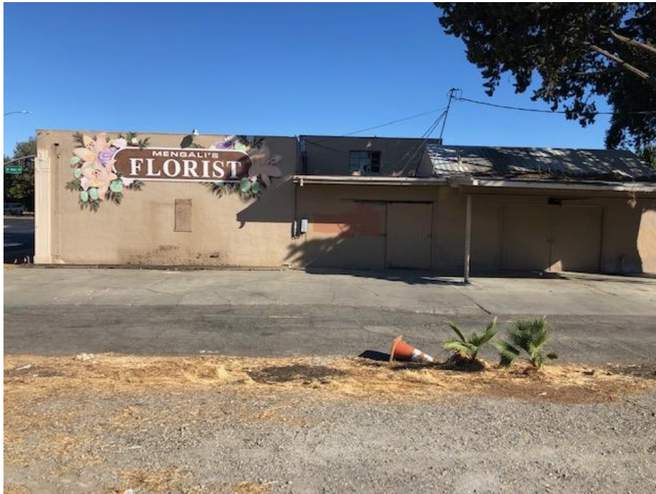
Photograph 5: View looking north at the rear or south elevation of 2 Main Street. Note the additions (right side) to the rear of the building.
