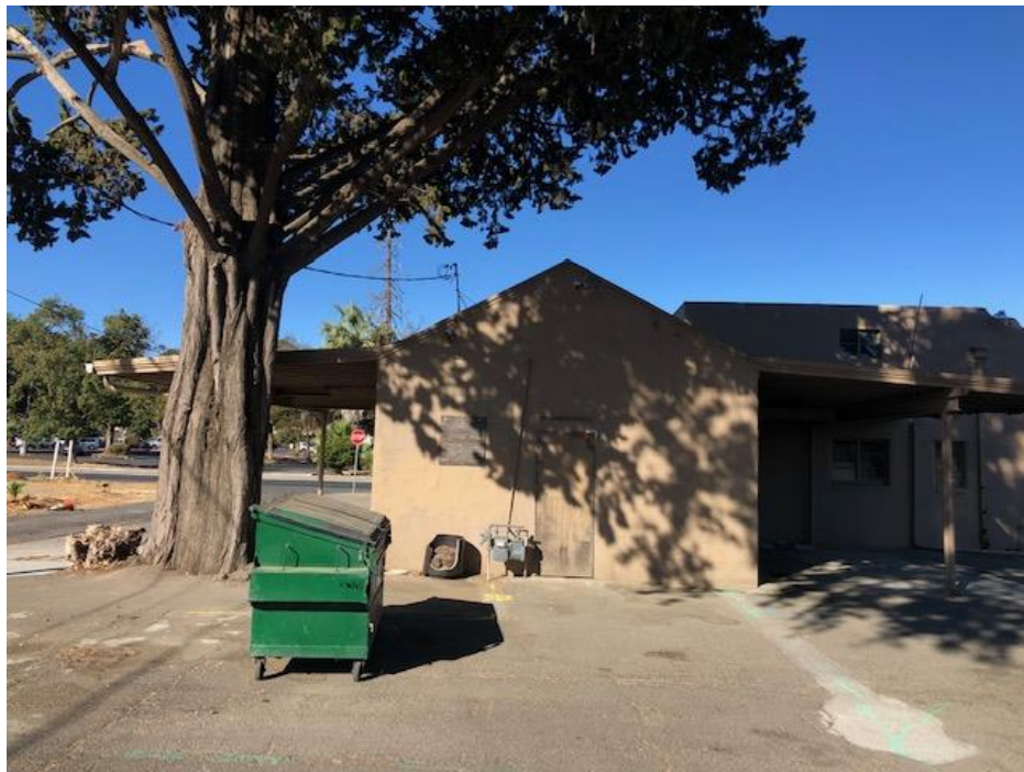
Photograph 6: View looking west at the east elevation of 2 Main Street illustrating the additions to the building.
