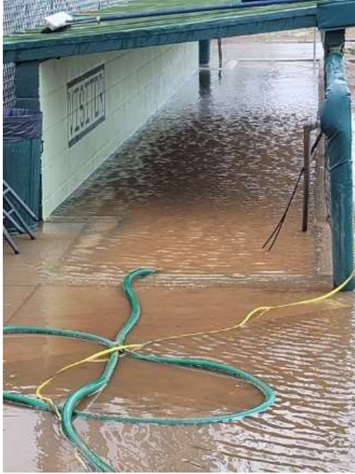
Clark Field dugout flooded with rain water
