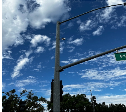
EVP GPS Antenna on signal mast arm shaft
