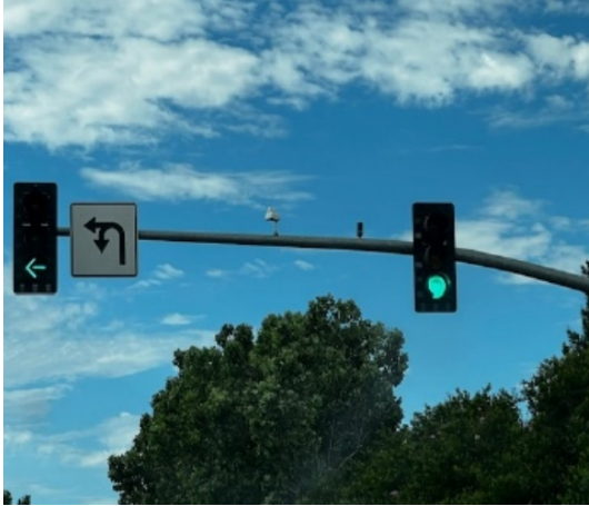
EVP GPS (White) Antenna with Inferred Detector on signal mast arm
