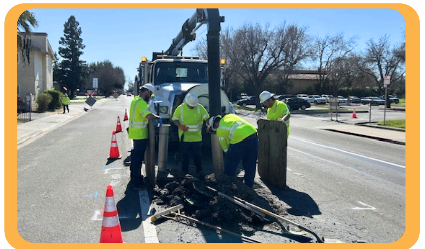
The Sewer Department hydro excavating for emergency repairs on the sewer lateral.
