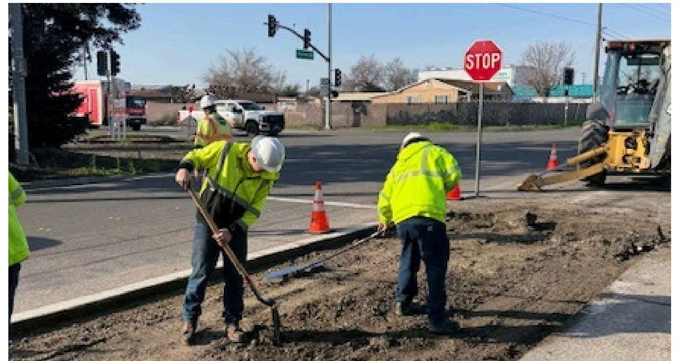
Streets Department crews remove damaged asphalt to prepare the roadway for smooth, durable repairs.
