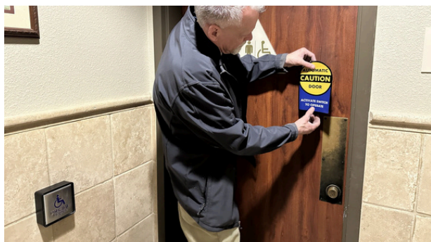
Automatic restroom door buttons installed at the Community & Senior Center.
