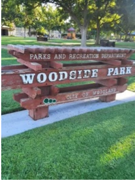
Woodside Park sign before repairs
