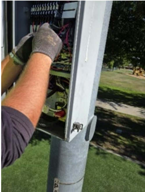
Capacitor installation at Woodland Sports Park
