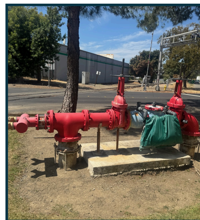
10 inch Fire Backflow.
